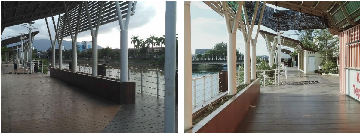
Figure 3. Condition of the Peunayong Riverwalk
