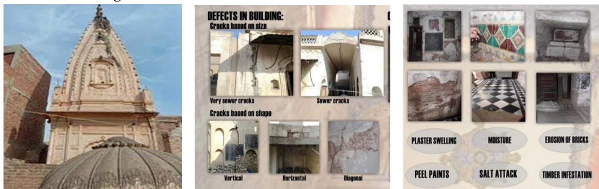
Figure 7. Existing defects in Temple building
